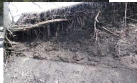
to determine the placement of each pin on the bank. The stream during peak flow created a noticeable line.
