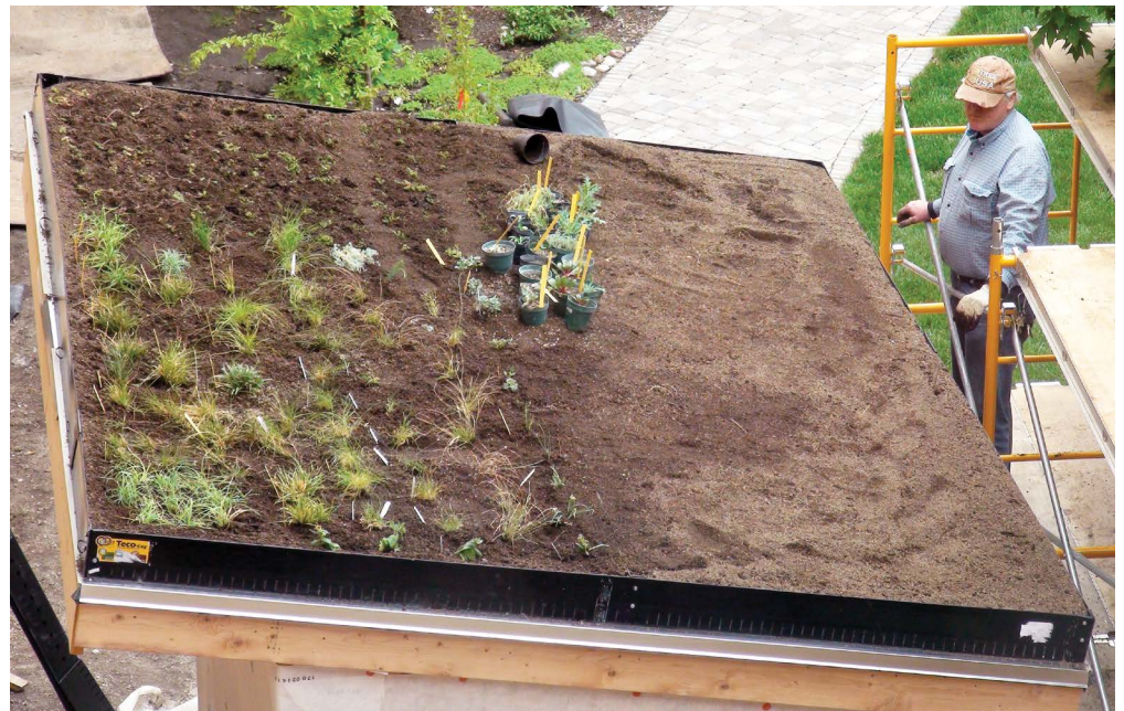
Dr. Richard Sutton inspects his work while constructing the green roof on the new outdoor cabinet in Keim Courtyard this spring.
